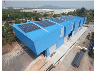
Solar power generation (Thailand: SYS)
