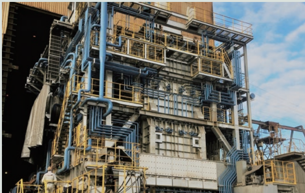
Single-stage furnace top scrap preheater (SSP)
